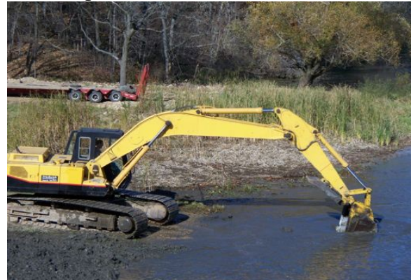
Friederick Excavating LLC removes accumulated sediments from the boat launch at Banfield County Park
